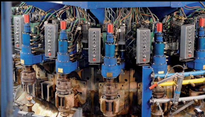
To increase capacity and flexibility in the production of top-quality glasses, the crystal factory in Amberg standardized the technology in its two production lines
